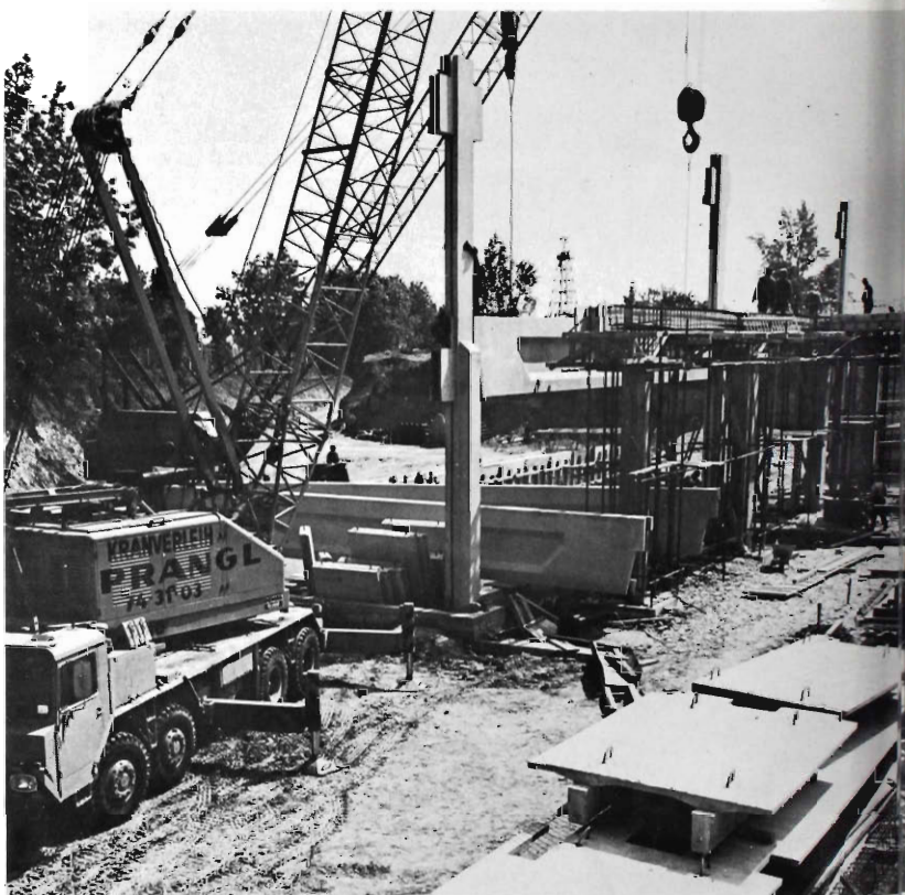
Fig. 9 To simplify construction most of the buildings in the Zentrum Wien complex utilized a system of reinforced-concrete girders and standardized supporting pillars which latch together somewhat like a giant erector set.
