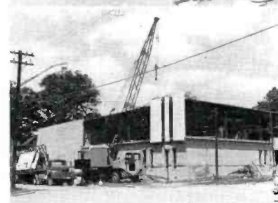
FIG. 4. Construction of new building started March 11, 1963 . . . by April 30 shell was erected and bricks laid . . . May 15 precast cement slabs arrived . . . During June and July equipment was installed . . . August 1 the station went on air!
