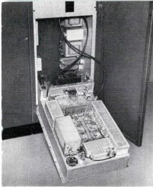
FIG. 3. Aural-visual exciter section of TTL-100AL/AH is easily tilted forward for servicing. Exciter is same type being used in many other RCA TV Transmitters, such as the TT-2BH, TT-6AL, and TT-25CL.
