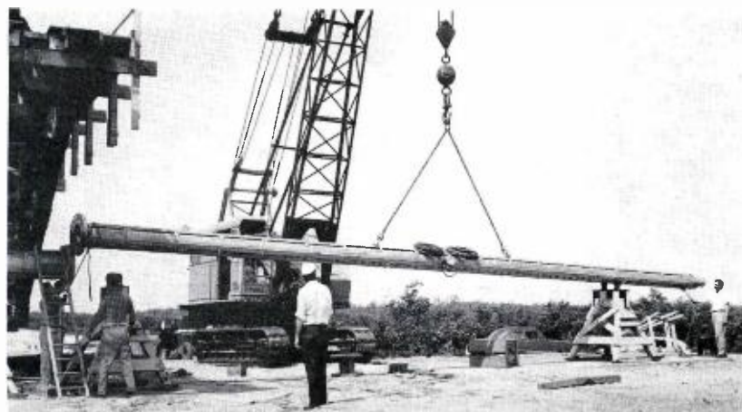
FIG. 7. Here two halves of a high-gain antenna are being assembled at the test site. Note crane which is part of normal equipment complement.
