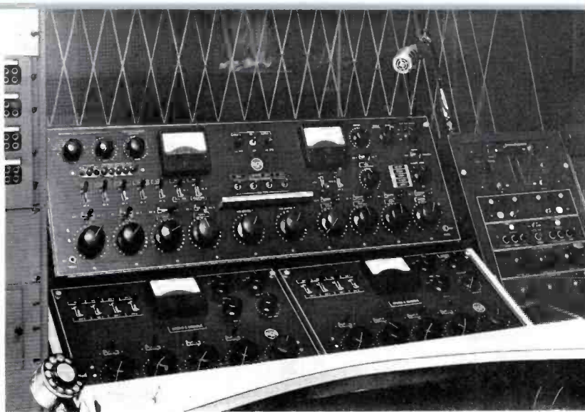
FIG. 4. Three consolettes are shown at the single operating position in the WCSH-TV control room. The BC-6A Consolette controls network, film and tape facilities, in addition to controlling the outputs of the two BC-5B Consolettes.
