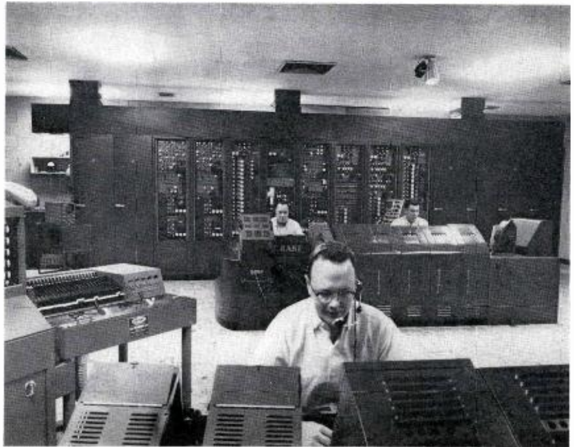
FIG. 15. Rack equipment behind master control: terminal equipment for audio and video; stabilizing and distribution amplifiers; and power supplies.
