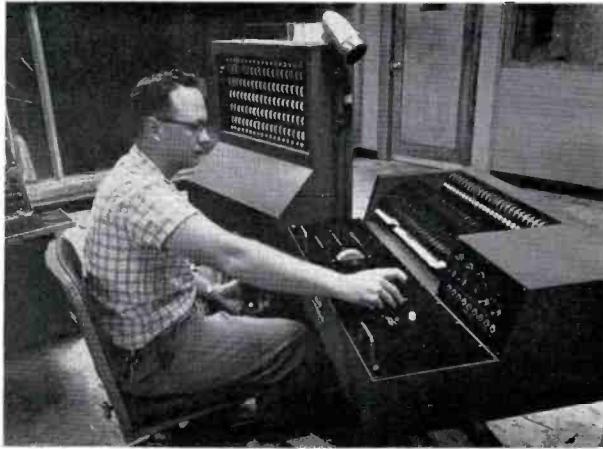
FIG. 9. Lighting control panel located in control room.
